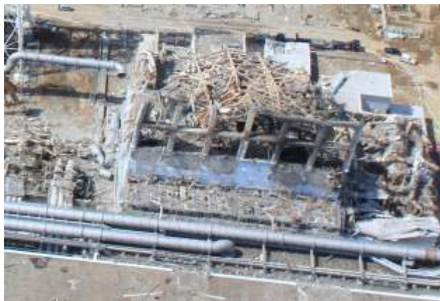
Reactor No. 3 (East side) Hydrogen built up in the 5 th & partially in the 4 th floor (north-east)
